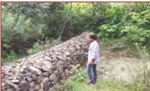
Loose Boulder Structure, Jharkhand
