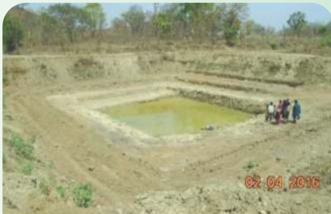
Creation of Water harvesting structure in Watershed area at Gola under IWMP project
